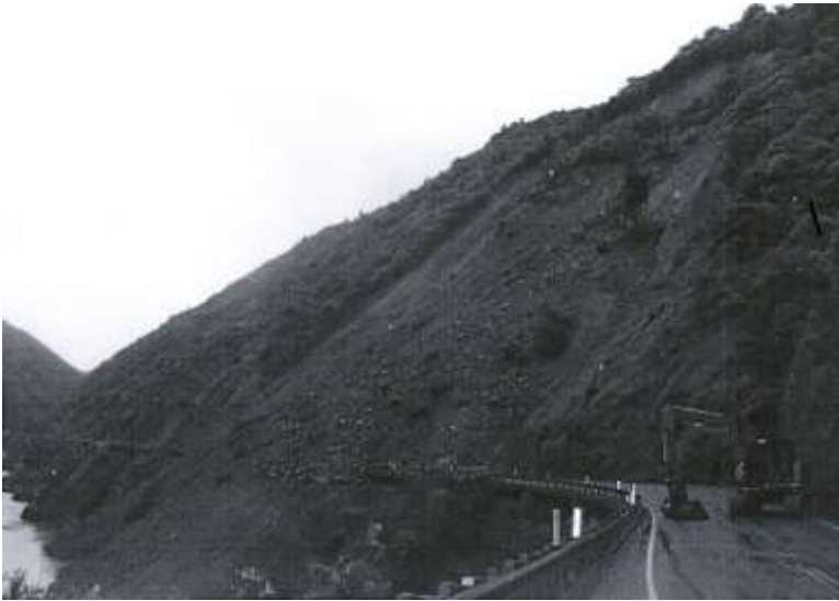
Massive Landslide during Winter flooding 2011 blocking main arterial route between Palmerston North and Napier
